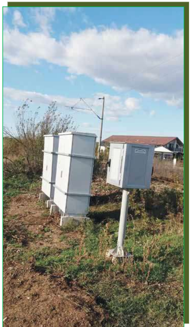
Dulapuri noi instalate BAT
