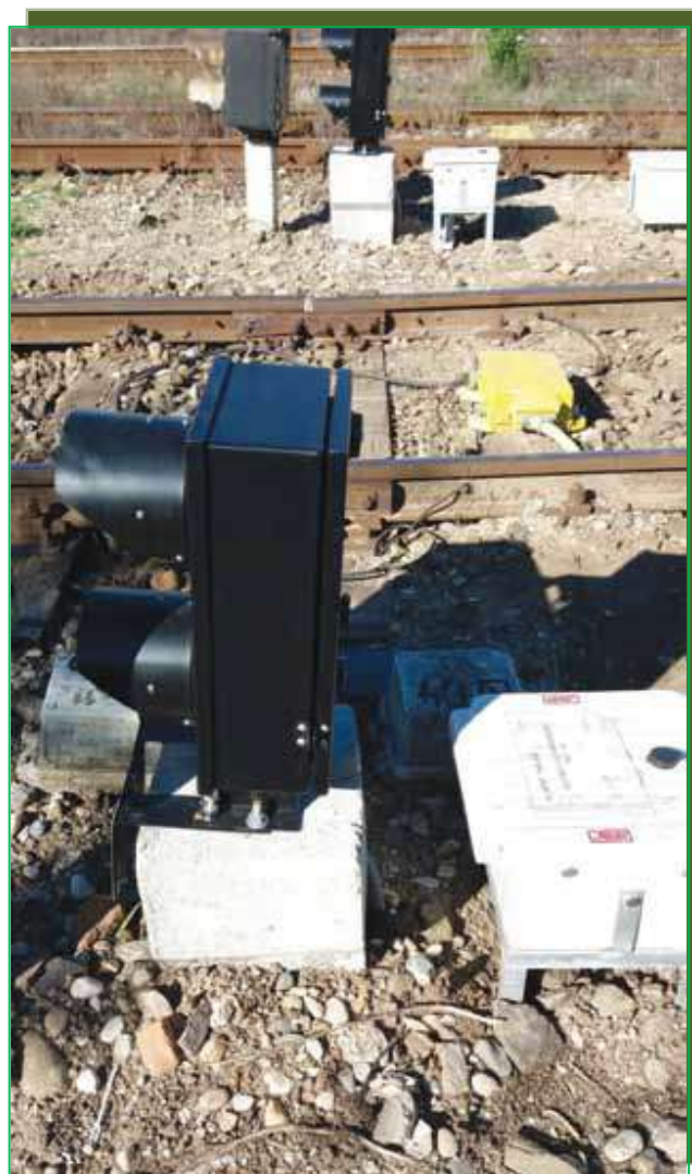
Echipament instalat: semnal manevra pitic, cutie aparataj
